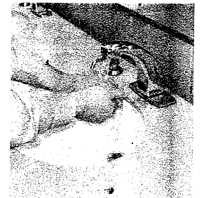
Figure 11.9 Some taps have touch or moisture detectors
