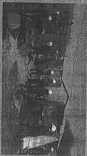
Habitat for Humanity volunteers helping to build a home for a beneficiary in Orange Farm, Gauteng.
