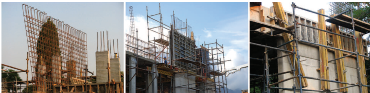
Figure 20: Steel reinforcement is put inside a concrete wall of a big building.
