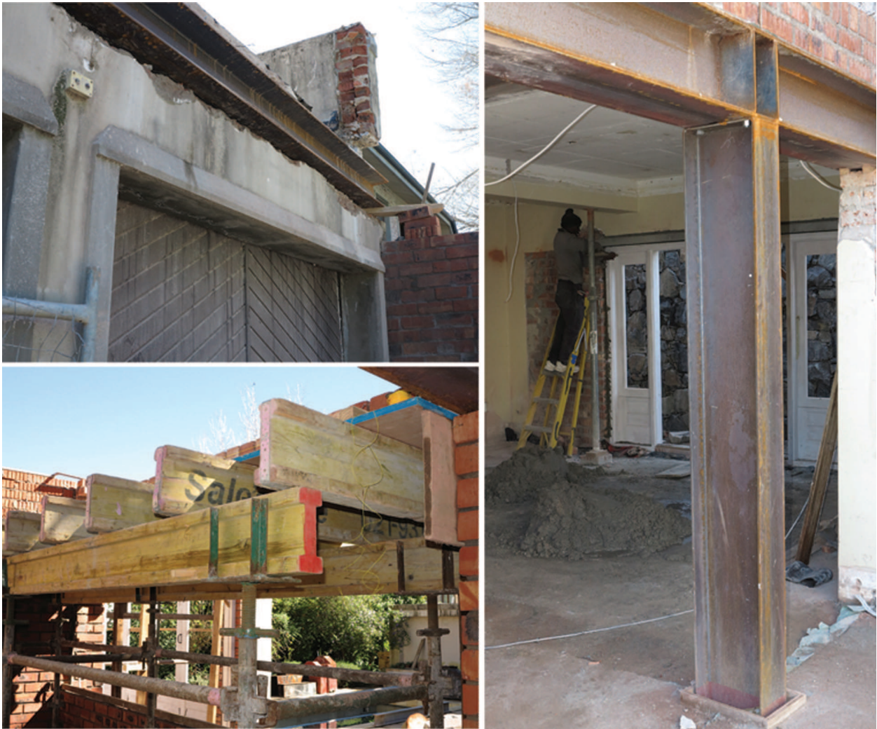
Figure 25: Steel I-beams are often used in buildings. Wood I-beams are often used during the construction of a building, but are removed once the building can support its own weight.
