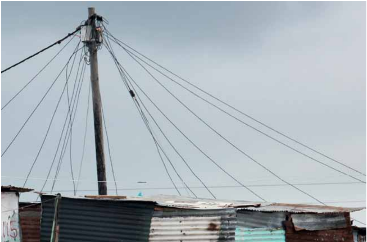
Figure 5: An informal community with an electrical supply. Notice the control boxes at the top of the poles. They control how much electricity each household uses and have a built-in safety mechanism for when there is a short circuit.
