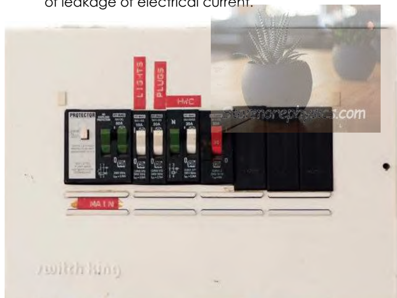
An electrical distribution board with circuit breakers
